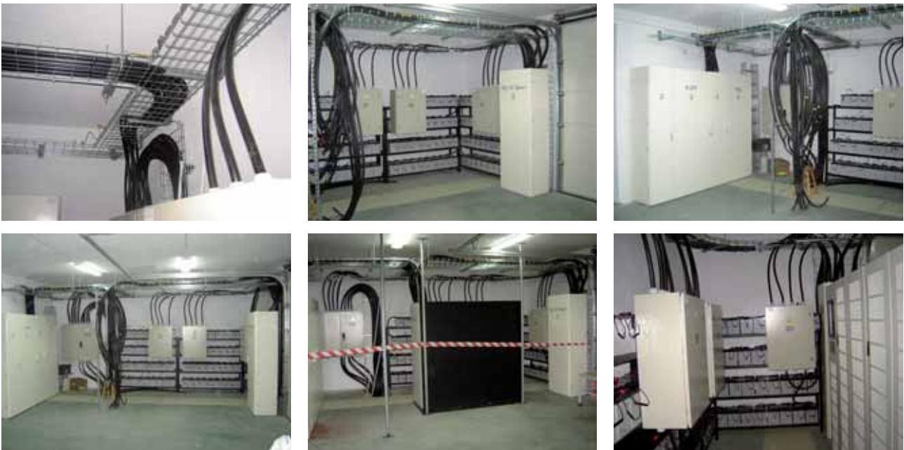
View of the uninterruptible power supply installation
